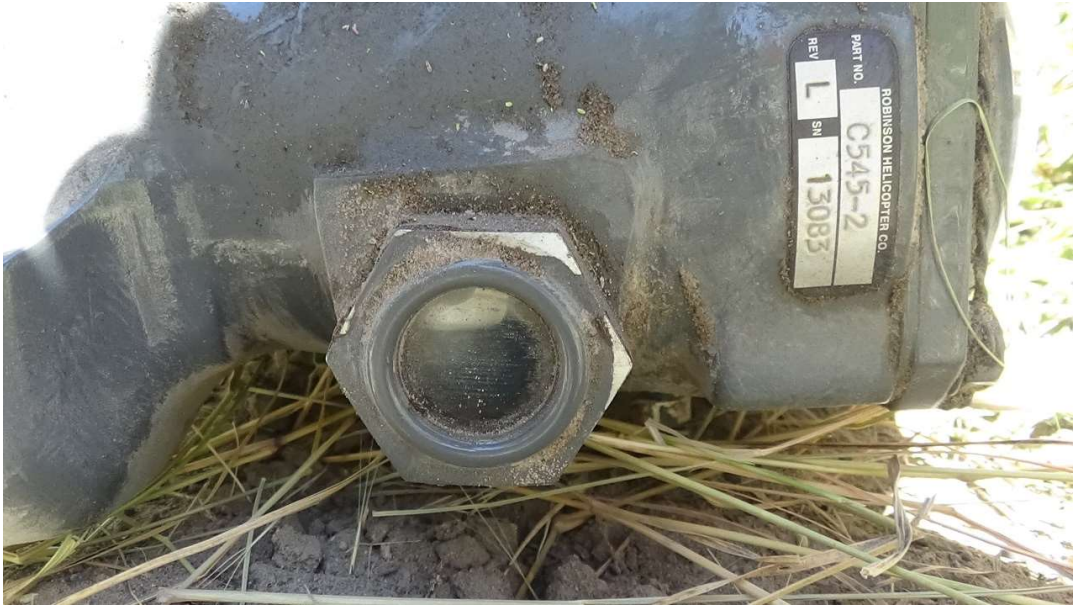
Figure 12c: View of the oil sight glass of the rotor gear-box.
