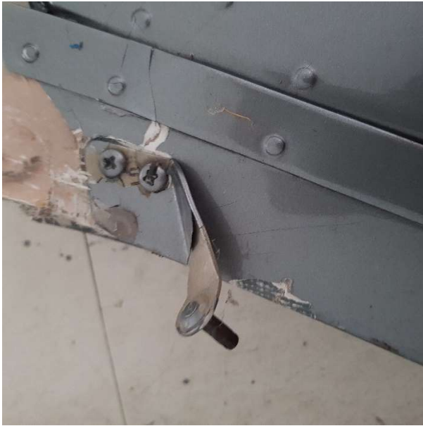
Figure 11c: Attachment component (lower door hinge) front left door.
